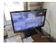
CCTV control room and monitors.jpg
